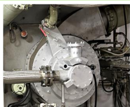
Ammonia burner as installed
