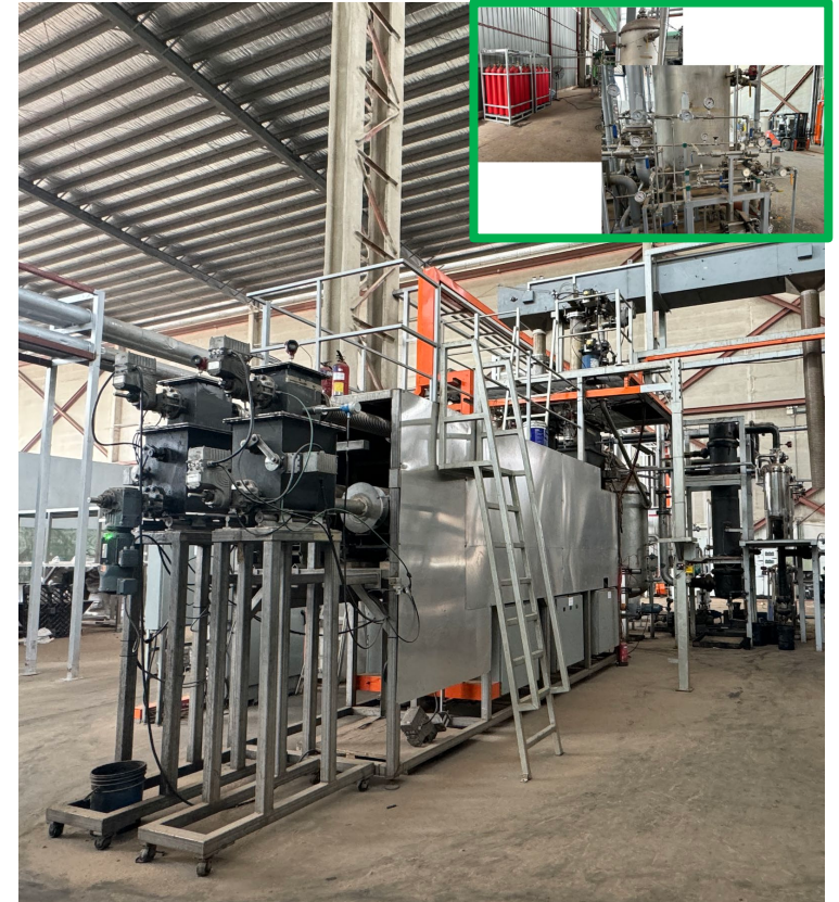
Above: GEIH Pilot Plant (Inset in green border: Syngas-hydrogen separation equipment)
