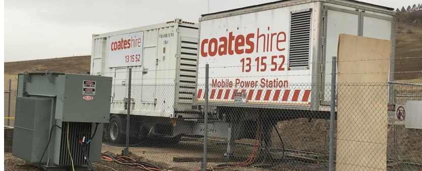
Genset deployed to Talbingo, NSW Snowy Mountains
