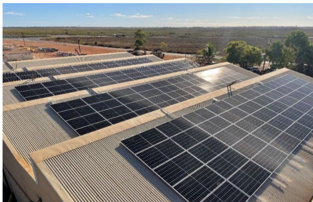
Newly installed Port Hedland solar panels
