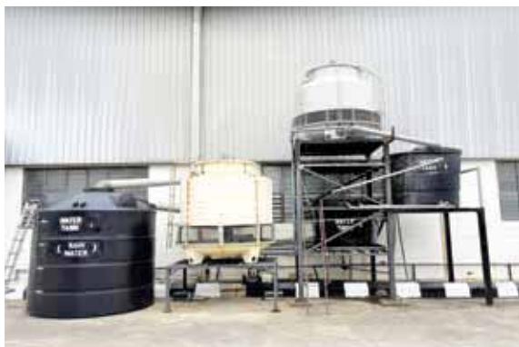
Cooling water system
