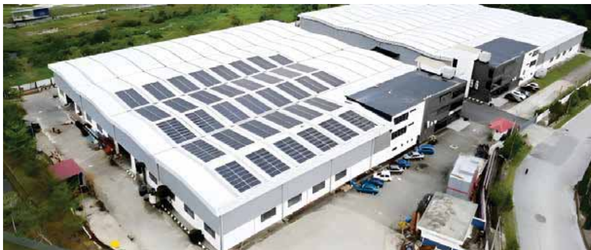
Solar PV Installation at Fibromat Rasa Facility
