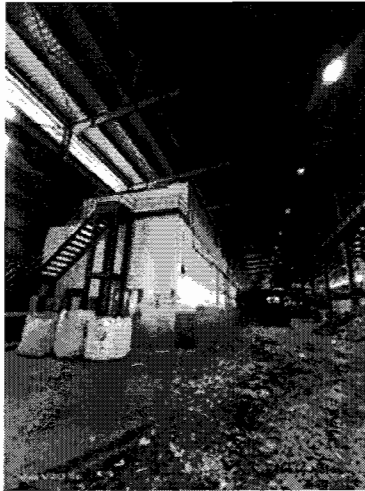
Washing Line Facility High Speed Pulp Separator.
