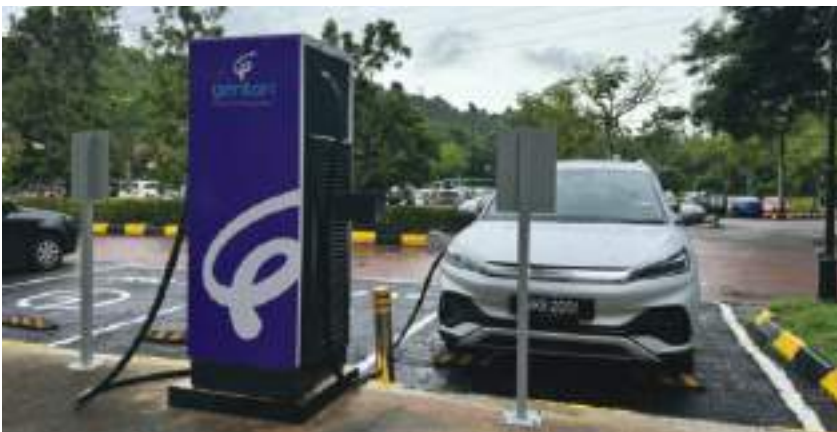
EV charging stations at Bukit Merah Laketown Resort
