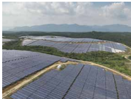
49MW Solar Photovoltaic Power Plant, Sungai Siput, Perak
