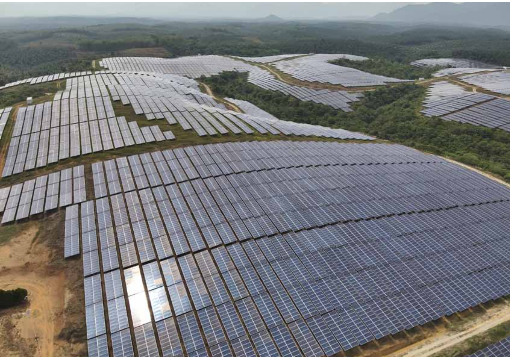
49MW Solar Photovoltaic Power Plant, Sungai Siput, Perak
