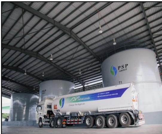
Our main warehouse at Lot 14827 consists of 3 silo tanks. Each silo tank is licensed to store up to 0.5 megalitre of diesel.
