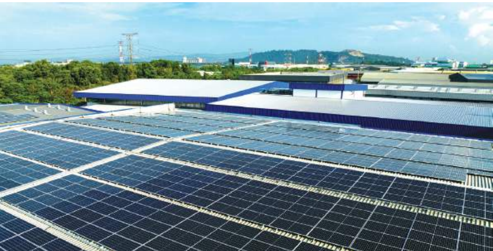
Solar PV system in Rapid Growth Technology Sdn. Bhd.
