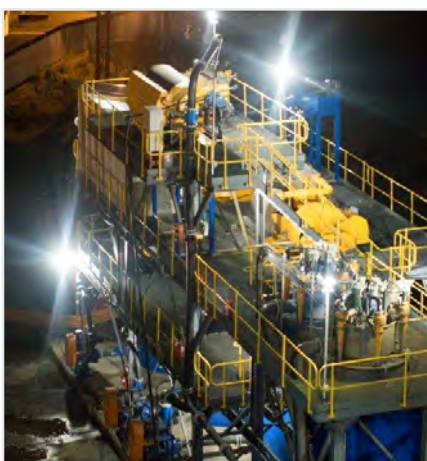
Figure 5 Fine chrome facility moved to Inyoni
