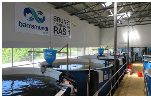
RAS tanks in Brunei are highly automated.
