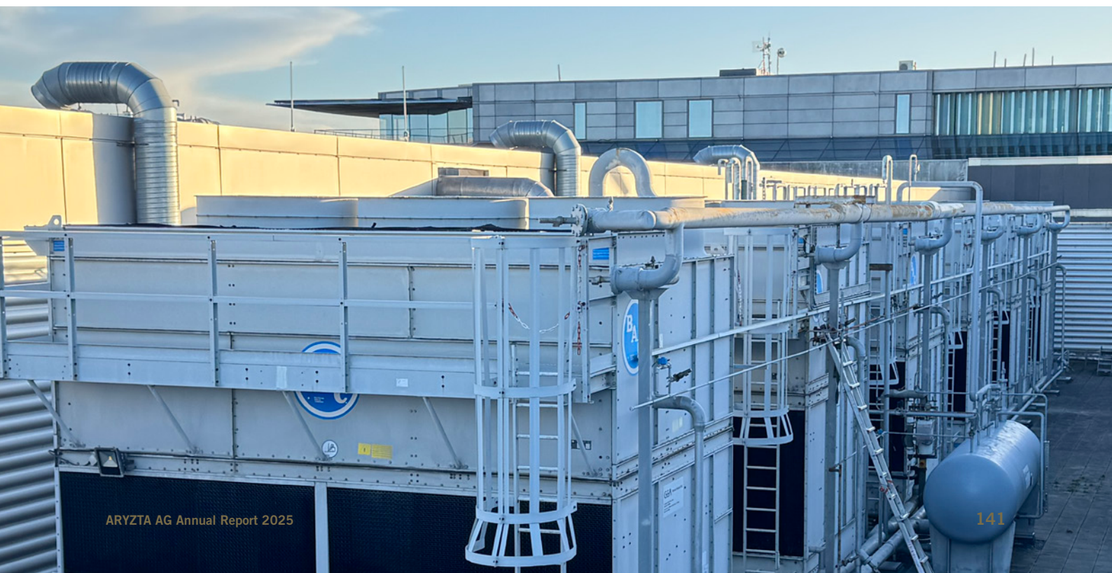
Condensers at ARYZTA Ireland
