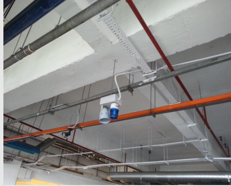
Panic Button Alarm System
