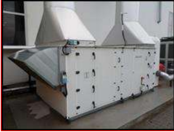
Klima Santrali AHU -1
